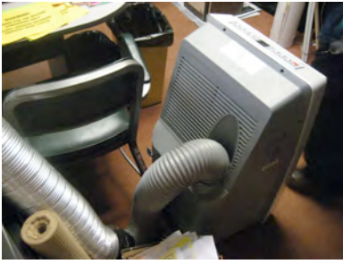
Portable Air Conditioning Unit
