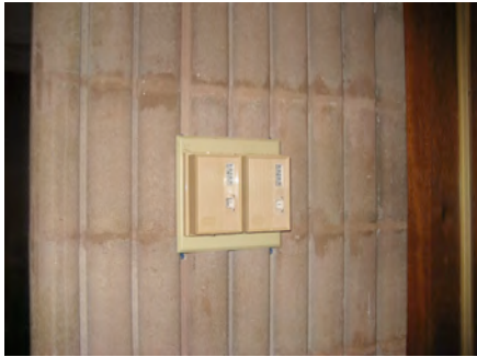
Manual Thermostats of old system
