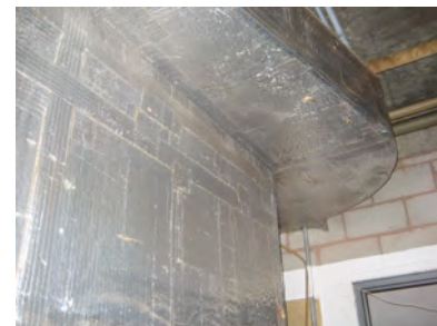
Air Ducts in Basement
