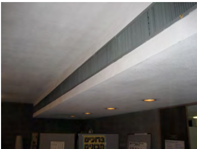
Air Ducts in the Sanctuary
