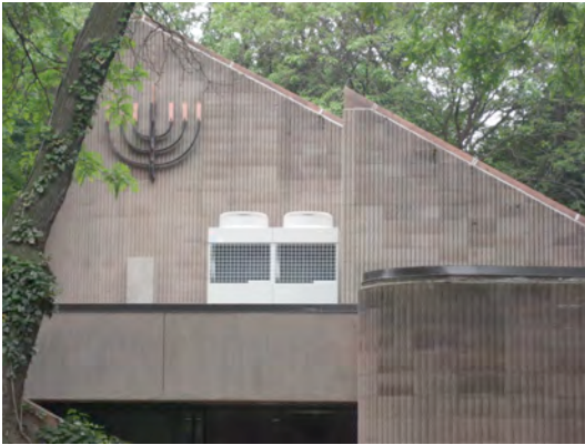
A view from the front of Boston Synagogue with the new Heat Pump
